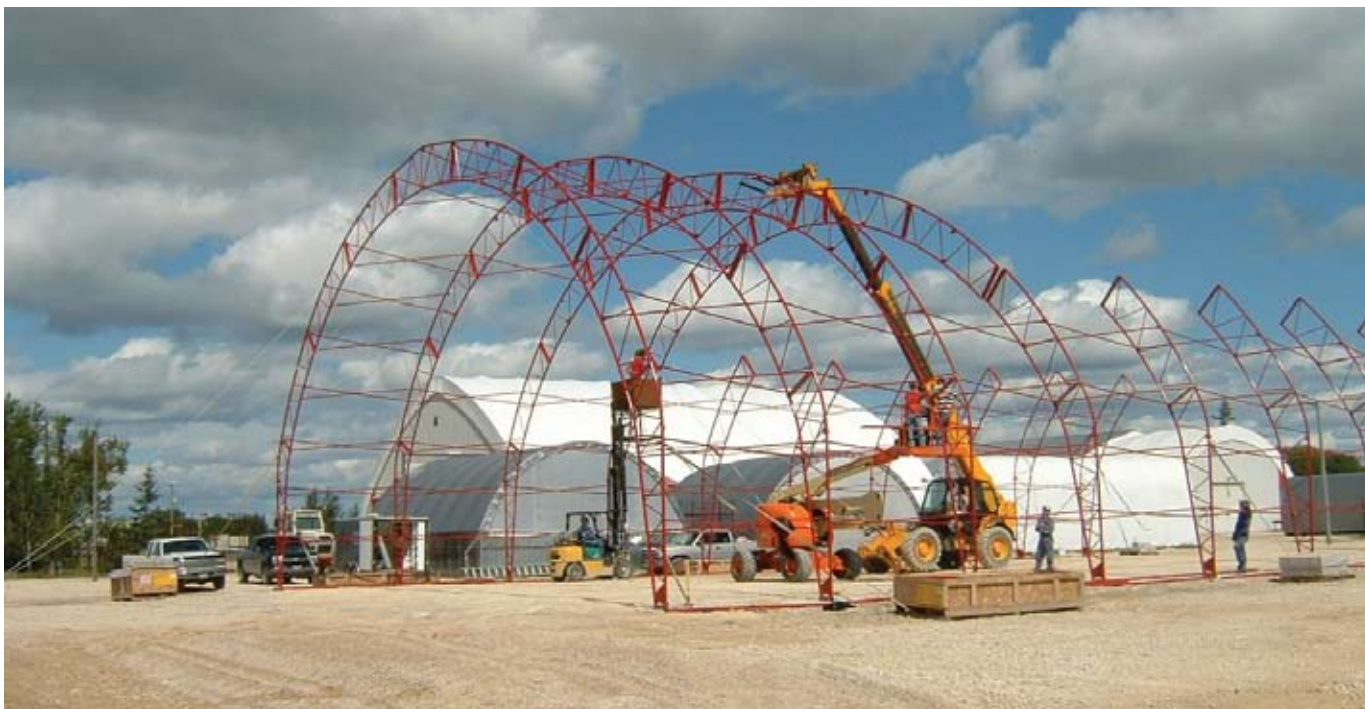
Last year Dueck Mechanical added 680 square metres of warehouse and yard space.
